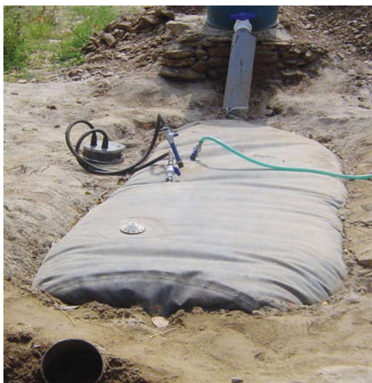
Fig. 2 : Flexible Balloon Stirring Digester at field (6 Cubic metre).
